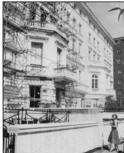
The ruin of the Iranian Embassy building as it stands today.
